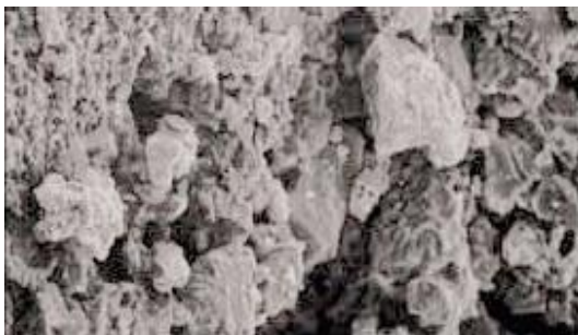
concrete without treatment
